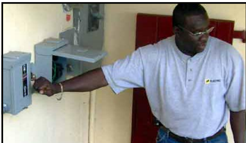
The Energy Office has helped many residents along on with projects that are capable of selling alternative energy back to WAPA. Above, Ira Francis, of NR Electric, is ready to throw the switch on at the home of Lloyd Williams on St. Thomas.
